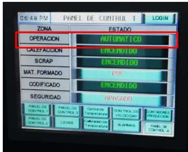
Figura. (7.2) 1: Panel de control Blistera #1 EEP-001-PD
