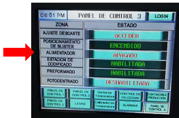
Figura. (7.7) 17: “Panel de control 3” blistera #1 SPS-300 EEP-001-PD.
