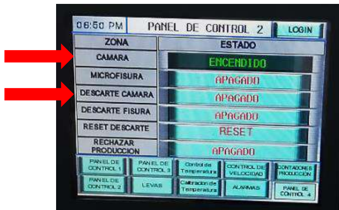
Figura. (7.11) 3: “Panel de control 2” blistera #1 SPS-300 EEP-001-PD.
